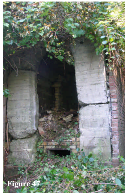
Figure 47: Concrete and brick structure near furnace stack to the east of the furnace. Perhaps associated with the Copake Plow Works.
